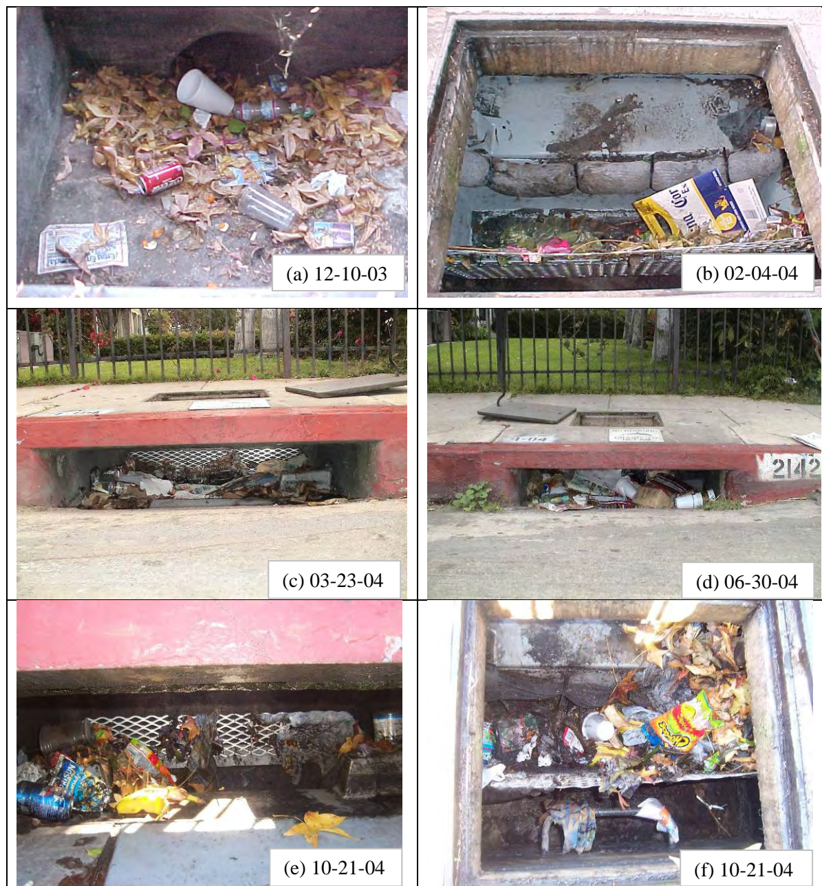
Figure 4-8. Field inspection photos showing the condition of Curb-Inlet Basket at the intersection of 23rd St. and Portland (east side).
