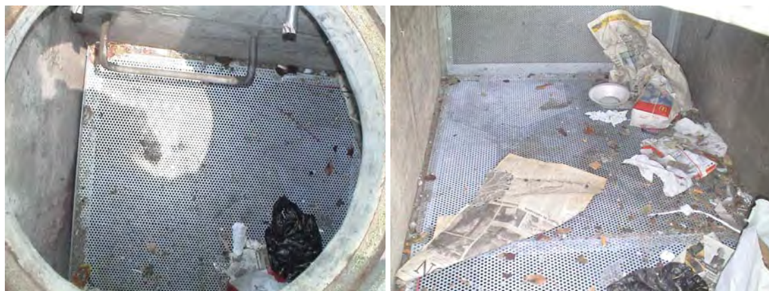
Figure 3-5. Alternative catch basin insert system installed by the City of Los Angeles.
