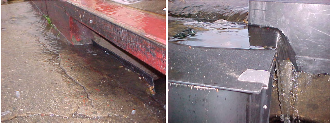
Figure 4-17. Relatively low-intensity storm showing bypass (FL-006-H, 2/4/04).
