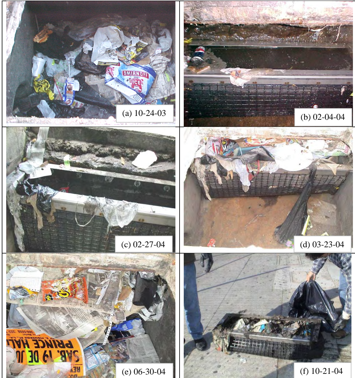
Figure 4-4. Field inspection photos of DrainPac catch basin insert at the intersection of Washington Blvd. and Vermont Ave.
