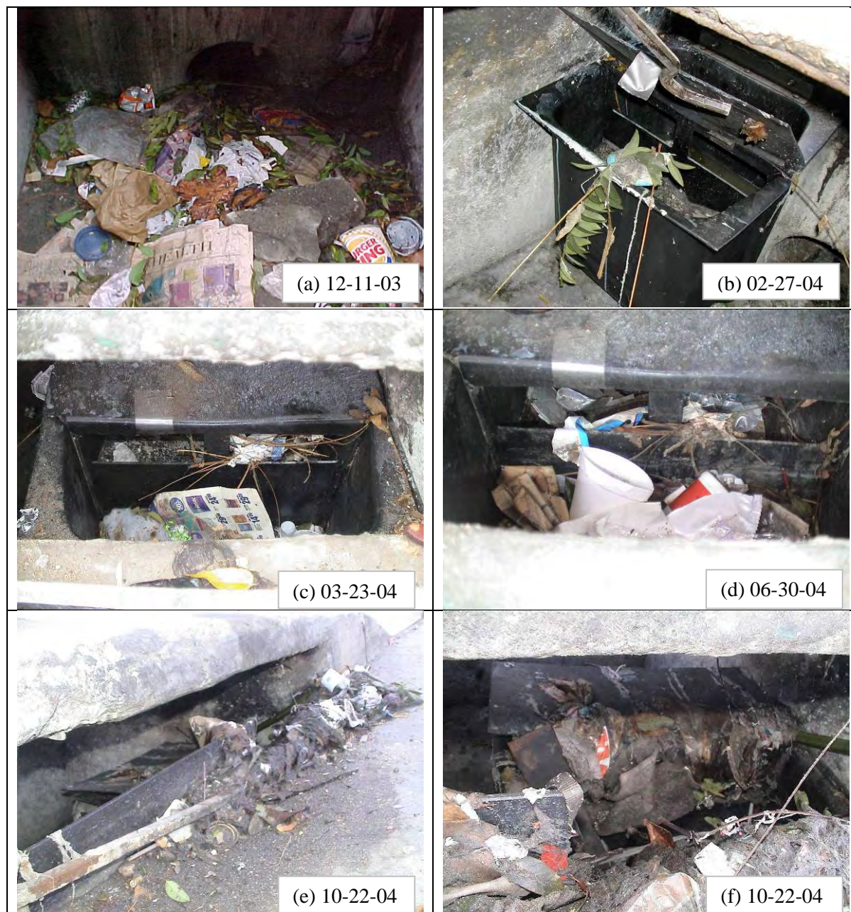
Figure 4-16. Field inspection photos showing the condition of Hydro-Kleen at the intersection of Washington and Walton.
