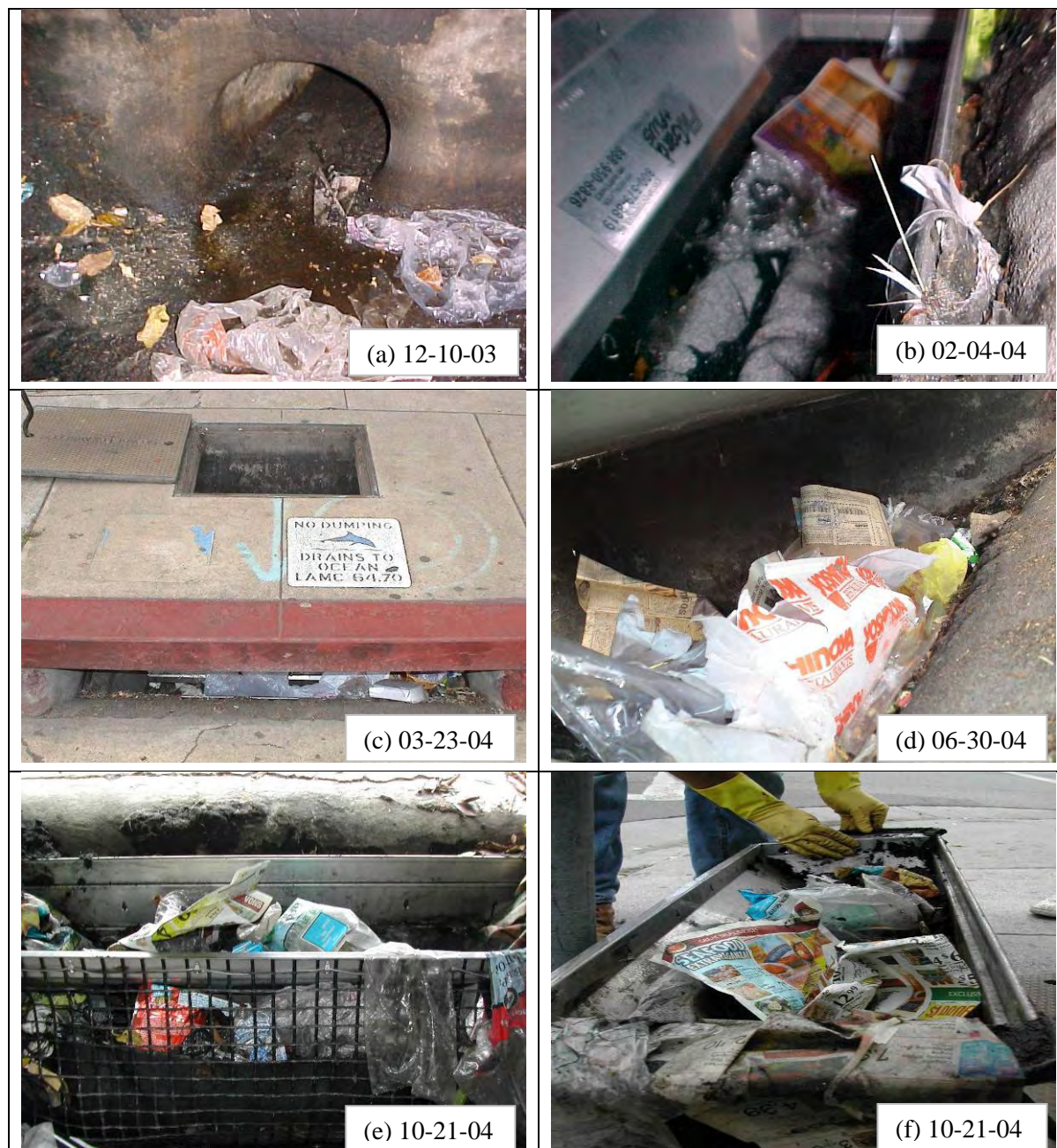
Figure 4-12. Field inspection photos showing the condition of FloGard Plus at the intersection of 18th St. and Flower St. (southwest corner).
