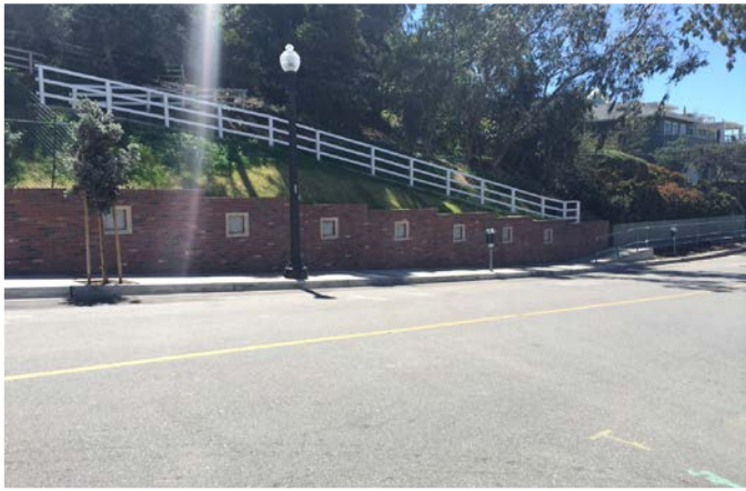
MERMAID STREET RETAINING WALL REPLACEMENT AND STREET IMPROVEMENTS CITY OF LAGUNA BEACH
