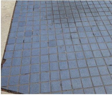
Figures 7.19 The current tile paving has failed in many locations and should be replaced
