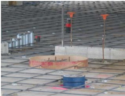
Above: The base for the fire pole from the fire residence area to the fire equipment.
