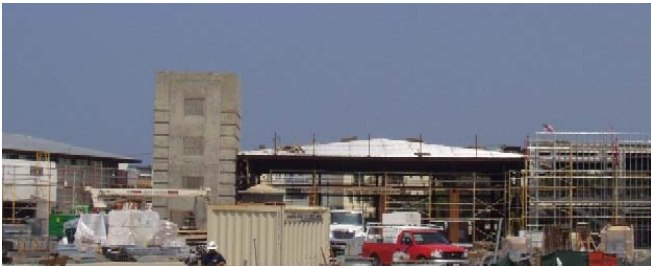
Above: All pours for the hose tower are complete. The tower will be finished this month.
