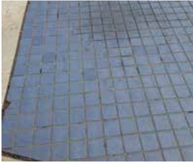
Figures 2-36 The current tile paving has failed in many locations and should be replaced
