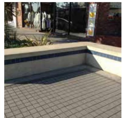
-F3 The concrete benches are worn and the inlay tile motif will need to be replaced to update this outdated look
