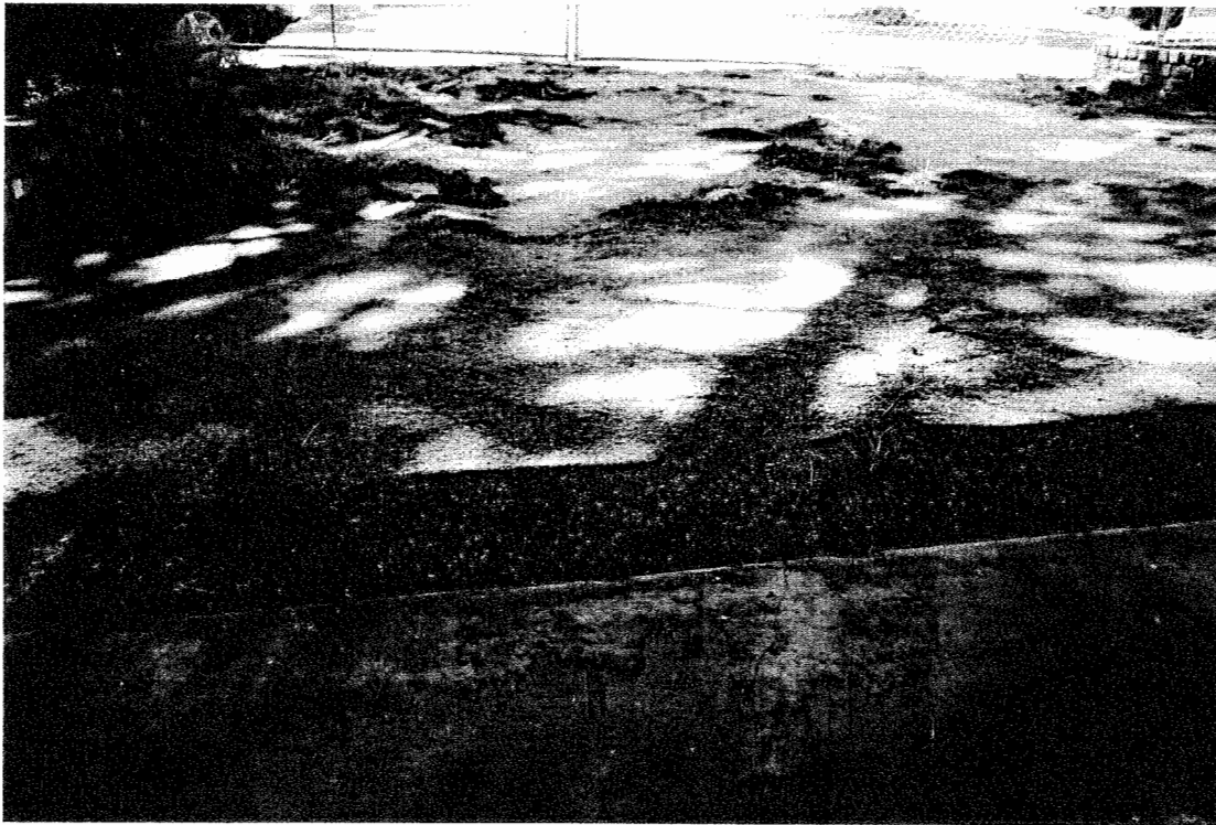
Pictures of damaged driveway
