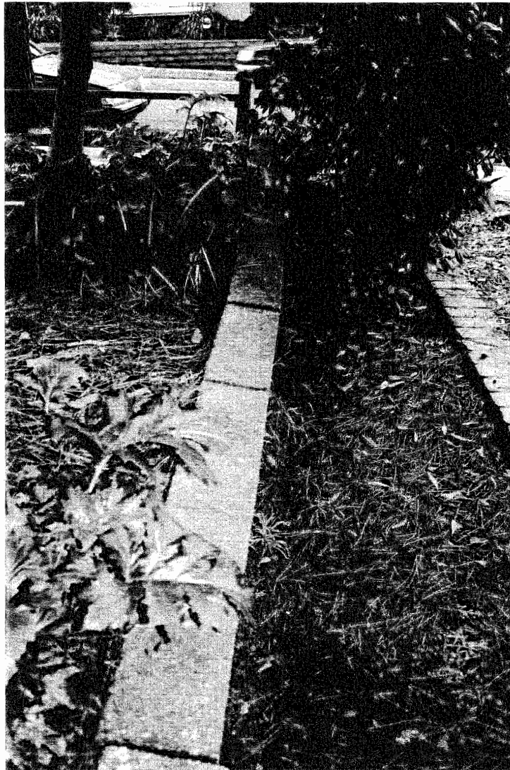
Damage to Retaining Wall
