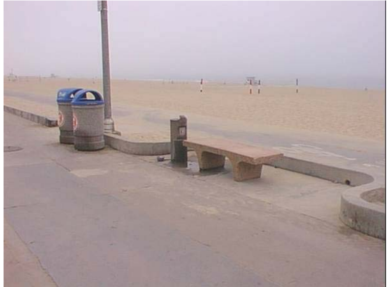
Typical existing bench and alcove. After the reconstruction, new trash receptacles will be placed in the alcoves instead of on the walkway as is depicted in this picture.
