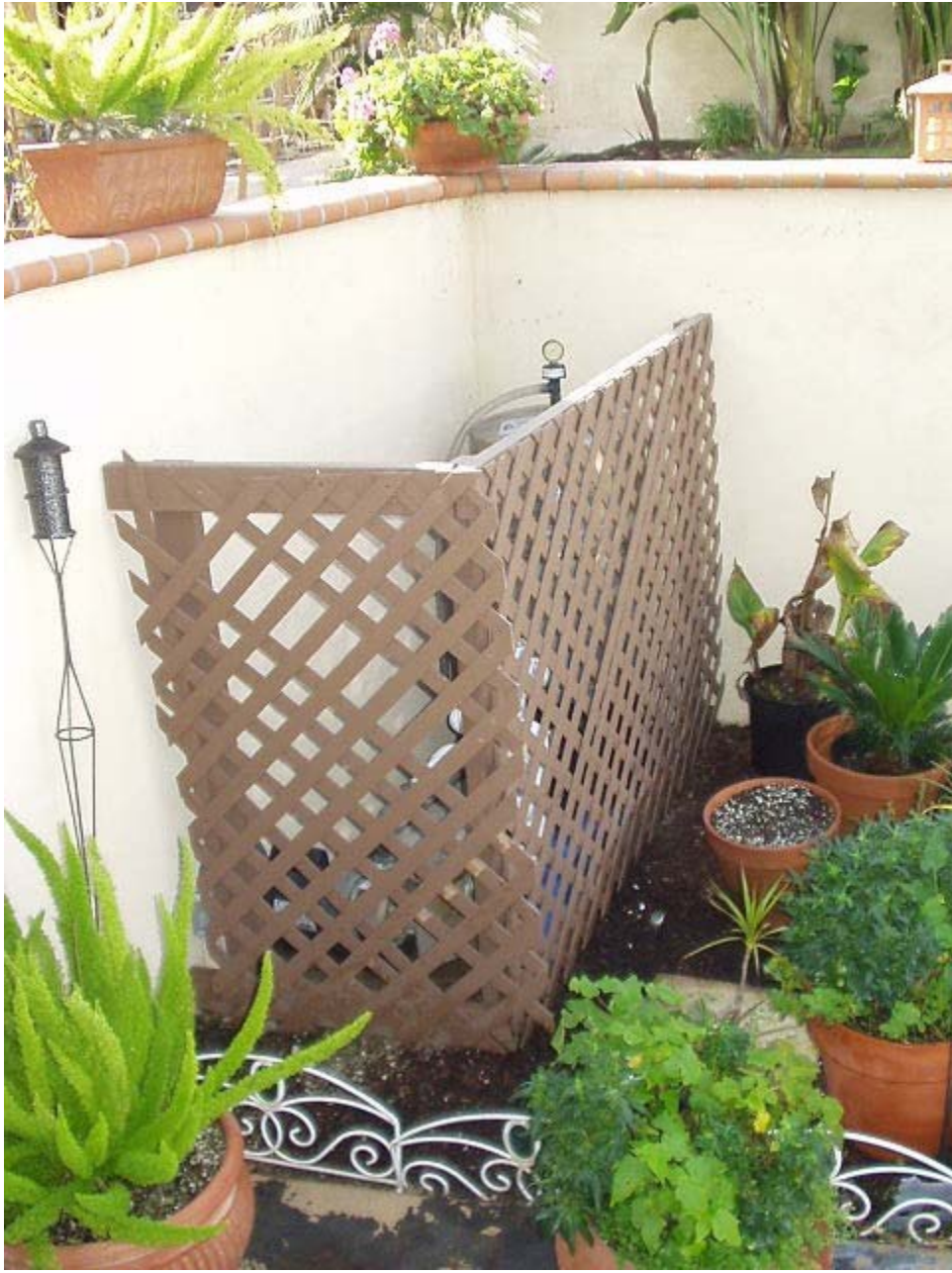
Existing Pool Equipment
