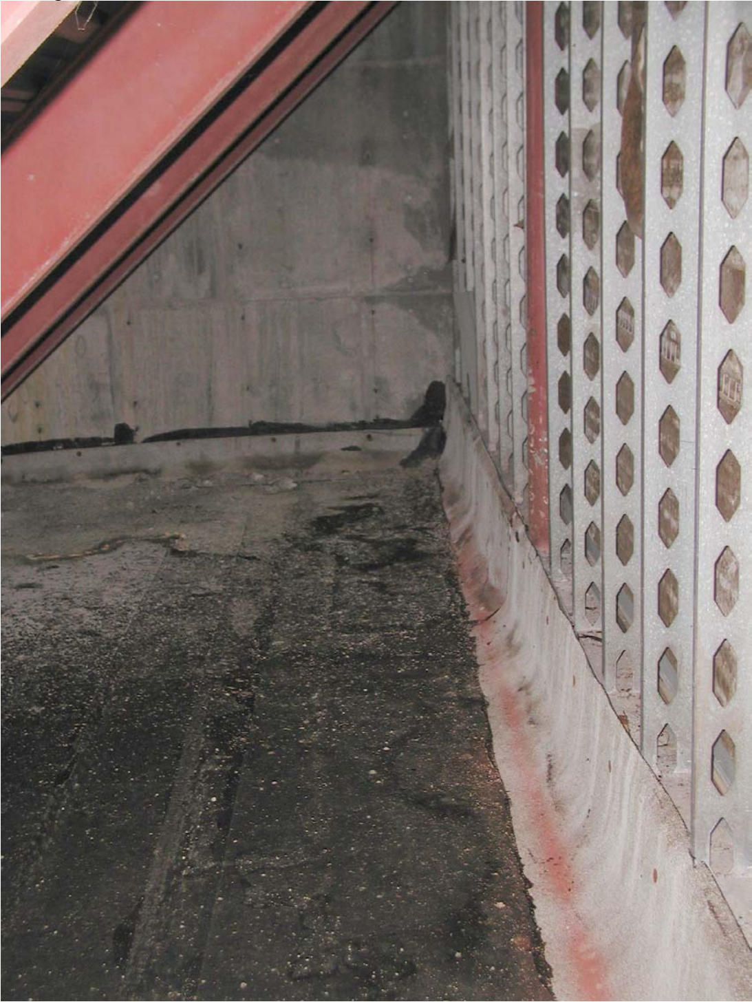
Damaged flat roof area.
