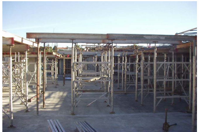
Above: The vast number of temporary elevated deck supports needed in preparation for pouring concrete
