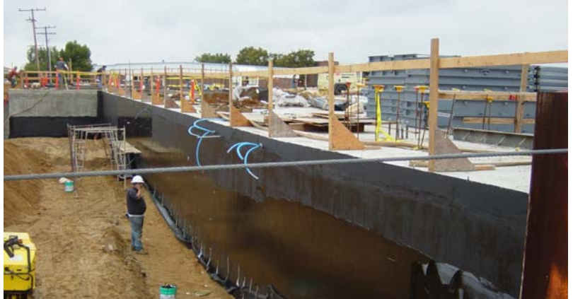
Above: Waterproofing the outer walls of the underground portion of the facility
