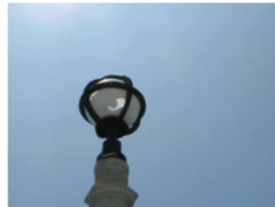
Damaged Pier Globe Lights
