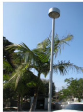
Parking Lot Lighting
