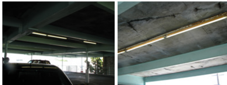
Dark Garage with Rusty Fixtures
