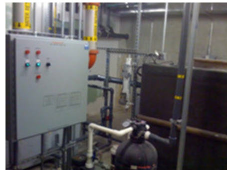
City Hall Mechanical Room
