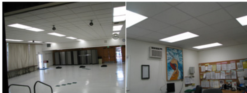
Joslyn Typical Lighting
