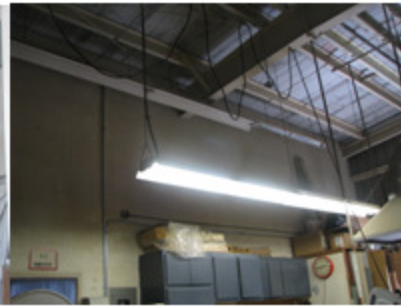
Suspended 8' T8 Fixtures
