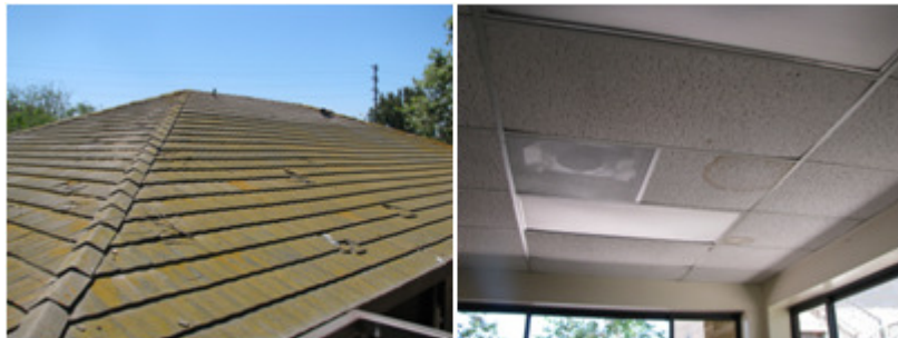
Roof Leaks due to Baseballs
