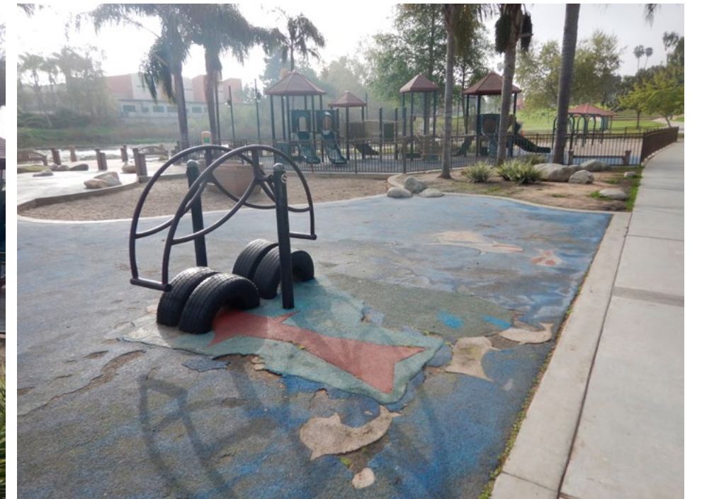
3. View from west of worn-out surfacing
