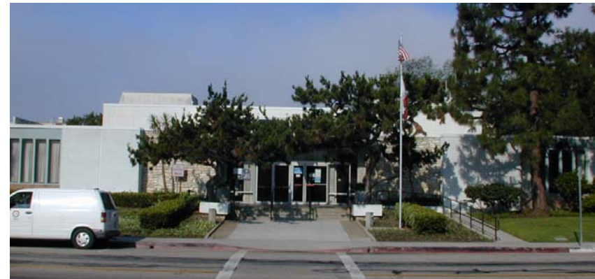
The Joslyn Hall. Built in the 1960s Joslyn Hall is an example of the state of community and recreation facilities in Manhattan Beach. Its structural, mechanical, electrical and plumbing systems have deteriorated, it violates building codes in almost every way and its size and configuration are inadequate for the delivery of programs and services the City provides.
