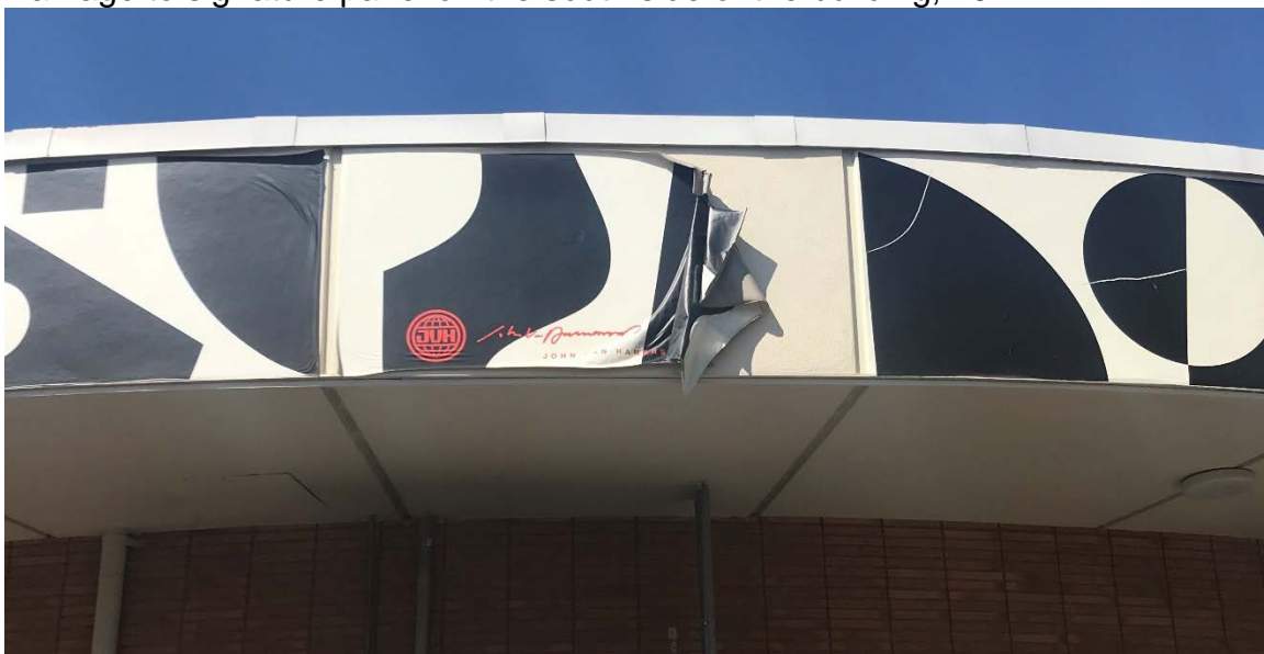
Damage to signature panel on the south side of the building, 2021
