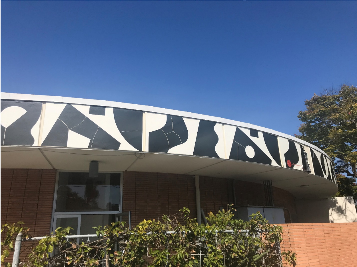
Cracks in black sections of the artwork, south side of building, 2021.
