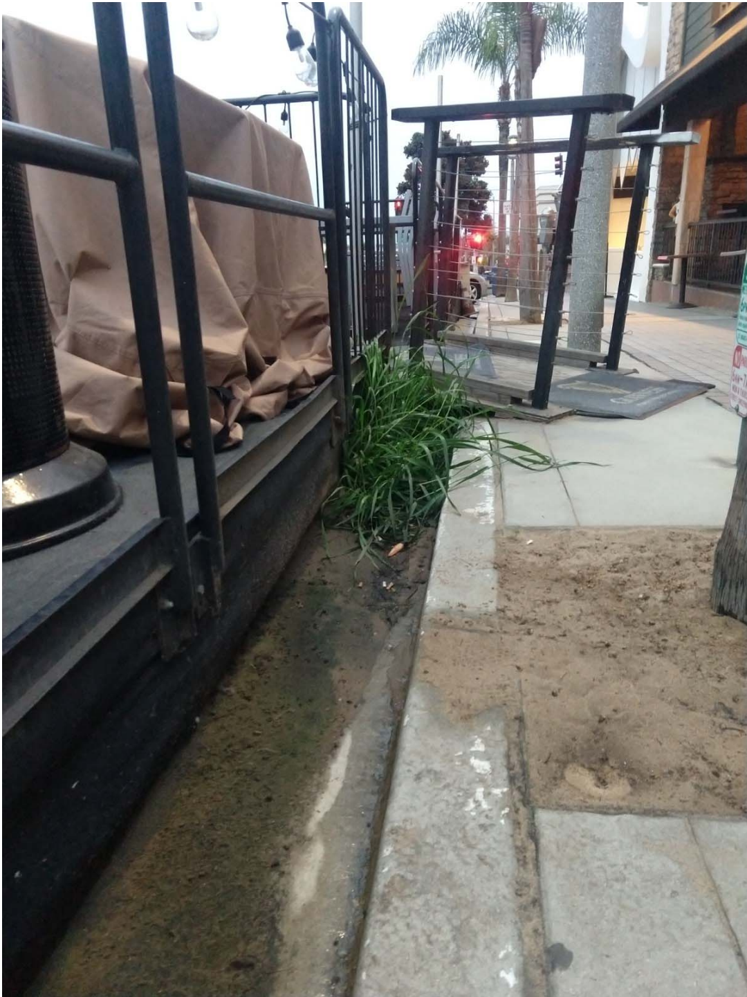
Sediment accumulation and vegetation growth due to Deck – stormdrain maintenance needed
