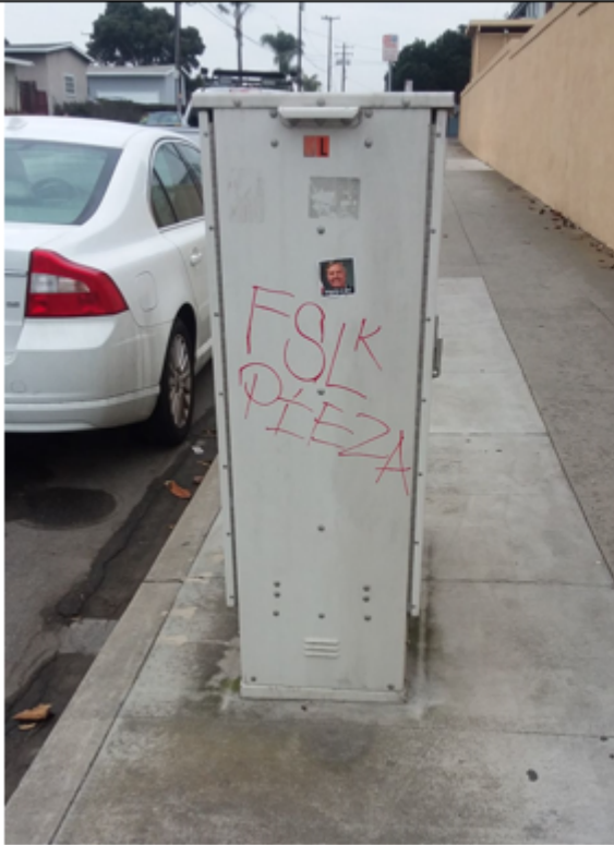
Graffiti, on electrical box, Tennyson Street
