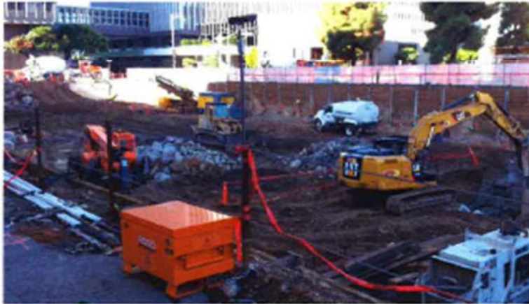
Figure 1: GEOVision vibration monitoring system at a DTLA site. Includes cellular remote email alarm and warning strobe.
