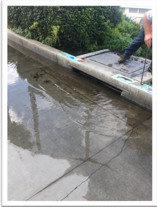
Photo #14 - Strand Stormwater Sump #11 at 43 rd Street
