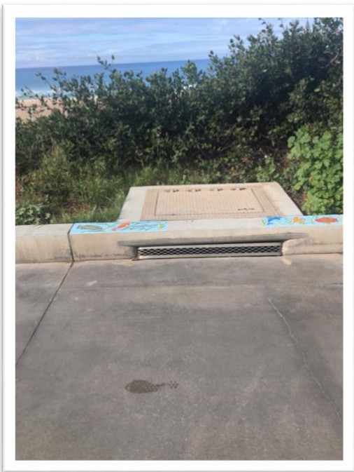
Photo #9 - Strand Stormwater Sump #8 at 28 th Street
