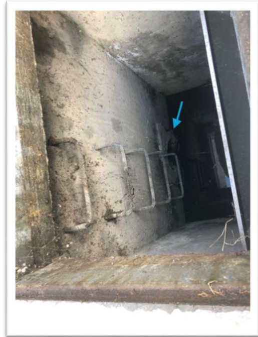
Photo #12 - Inside Strand Collection Basin #9 at 39 th Street – Note outlet pipe denoted by blue arrow which ties into MS4 outfall that discharges onto beach.
