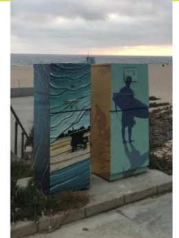
Wrapped Utility Boxes Hermosa Beach, CA
