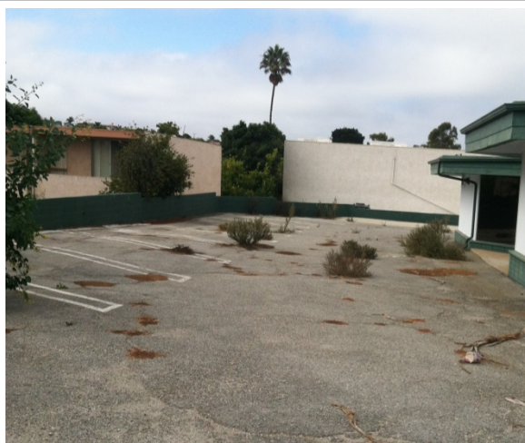
Vacant commercial property with significant deterioration.
