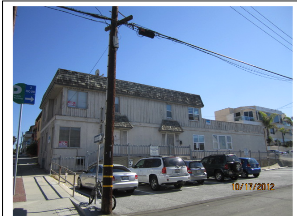
Older underutilized multi-family building showing signs of disrepair and vacancies.
