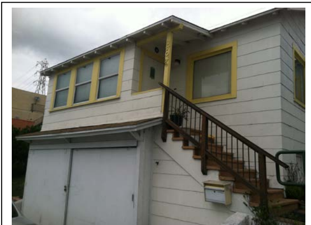
Older residential buildings showing disrepair, low site utilization and functional obsolescence.
