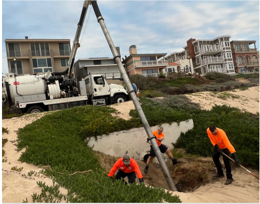
Crew vacuuming trash from storm drain outfall at the beach that was flushed down a storm drain pipe
