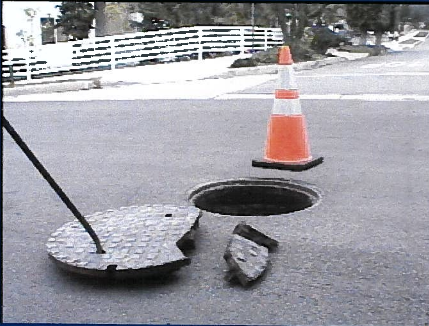
Broken Manhole Cover
