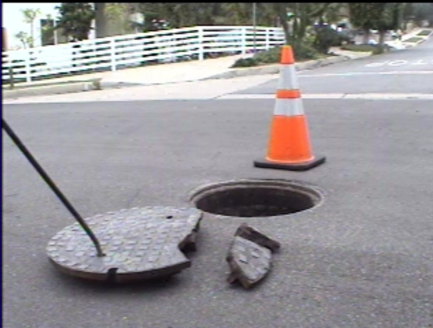
Broken Manhole Cover
