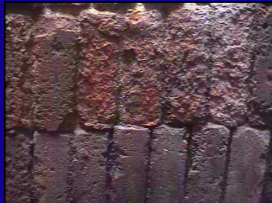
Corrosion in Manhole
