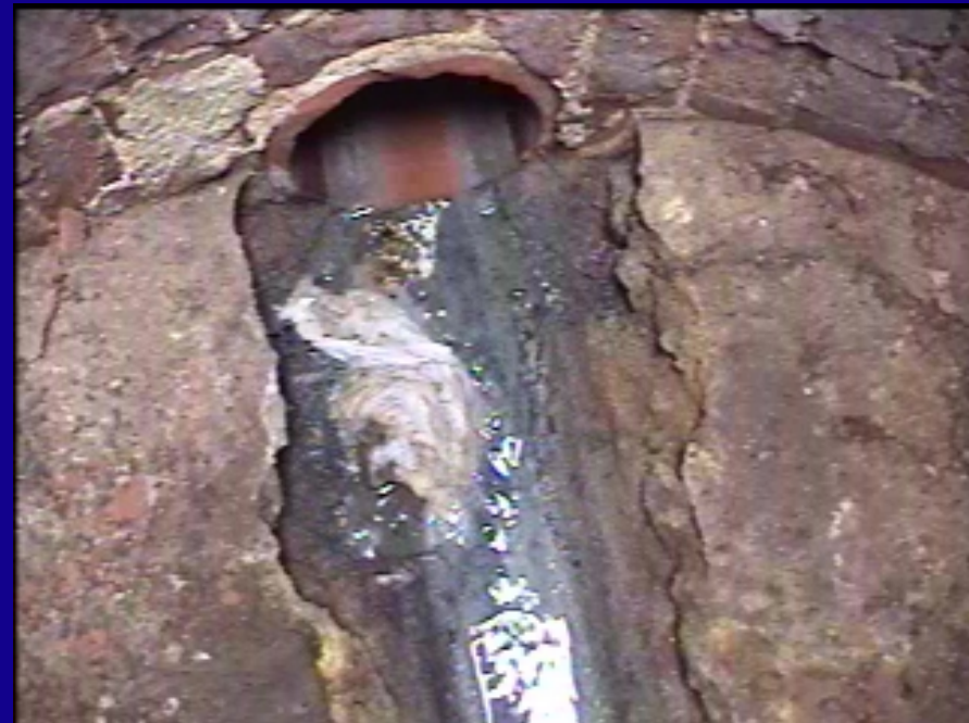
Eroding Channel in Manhole
