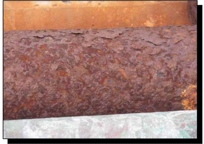
Photograph 6-33 Pier Pump Station Forcemain Close-up
