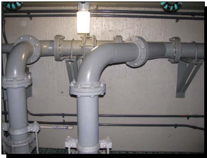
Photograph 6-21 Meadows Avenue Pump Station Discharge Header
