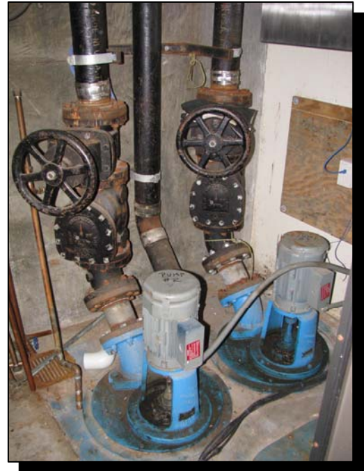
Photograph 6-29 Civic Center Pump Station Pumps
