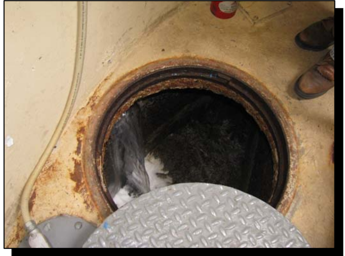
Photograph 6-16 Poinsettia Avenue Pump Station Wet Well
