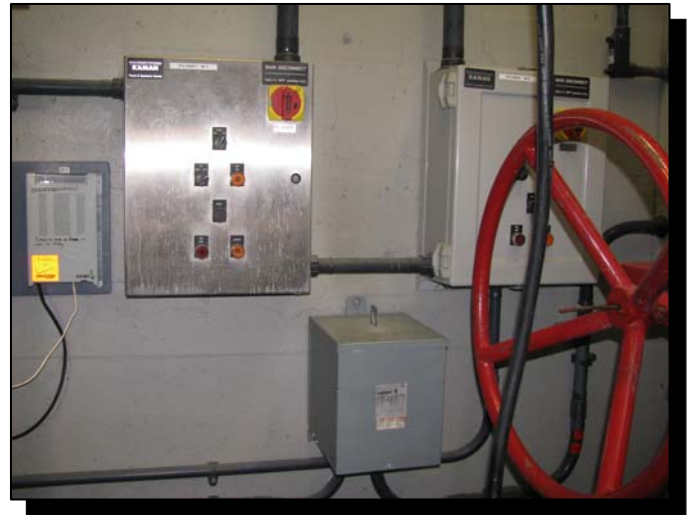
Photograph 6-5 Bell Avenue Pump Station Control Panel
