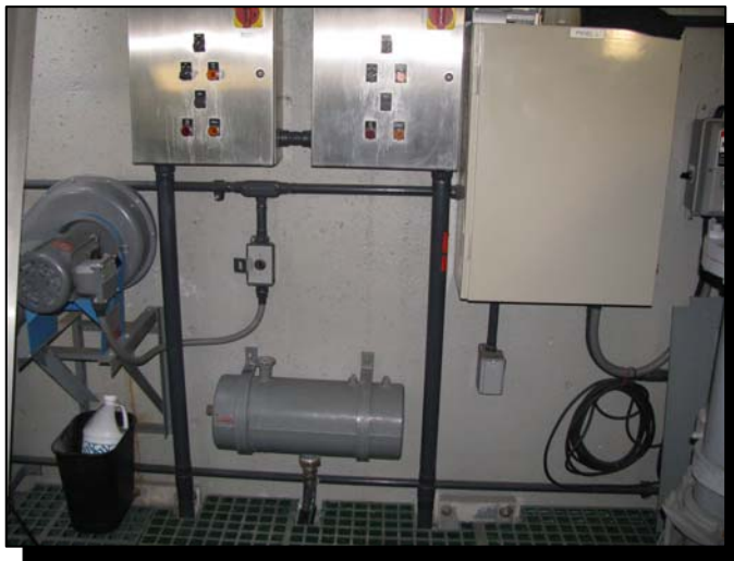
Photograph 6-23 Meadows Avenue Pump Station Control Panel
