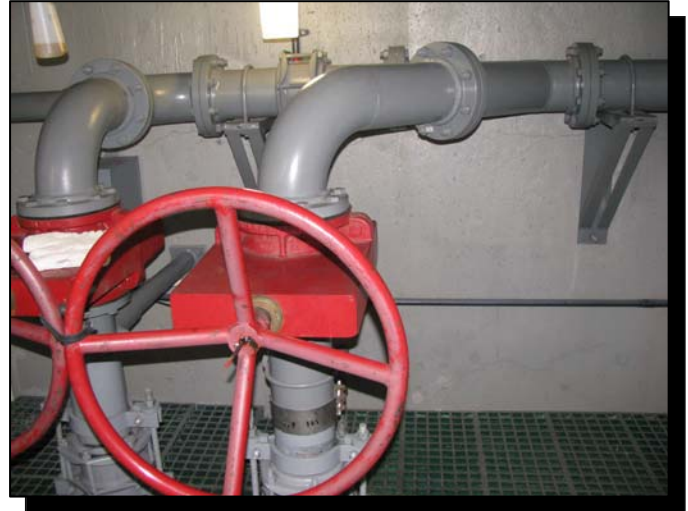
Photograph 6-13 Pacific Avenue Pump Station Discharge Header
