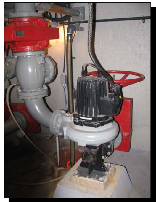
Photograph 6-26 Voorhees Avenue Pump Station Pumps
