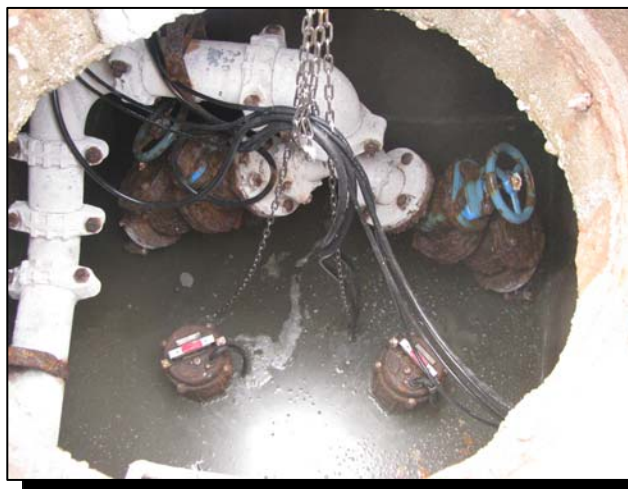
Photograph 6-31 Pier Pump Station Wet Well
