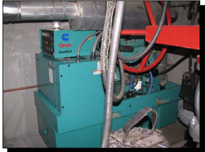
Photograph 6-10 Palm Avenue Pump Station Generator
