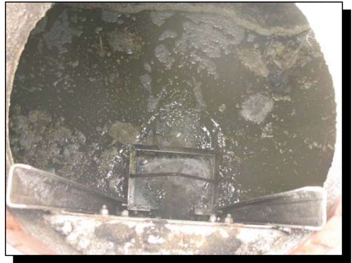
Photograph 6-7 Palm Avenue Pump Station Wet Well
