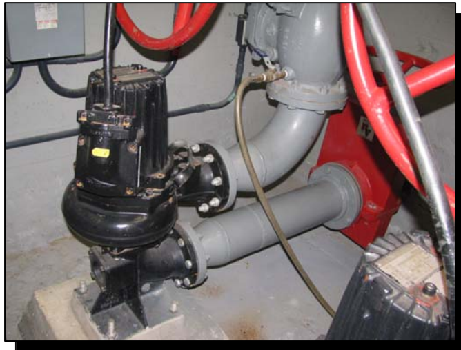
Photograph 6-4 Bell Avenue Pump Station Pumps
