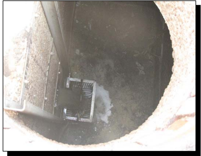
Photograph 6-20 Meadows Avenue Pump Station Wet Well
