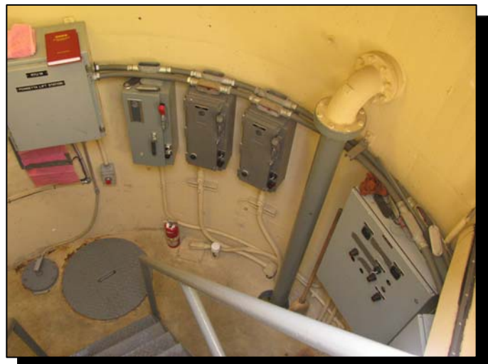
Photograph 6-18 Poinsettia Avenue Pump Station Control Panel
