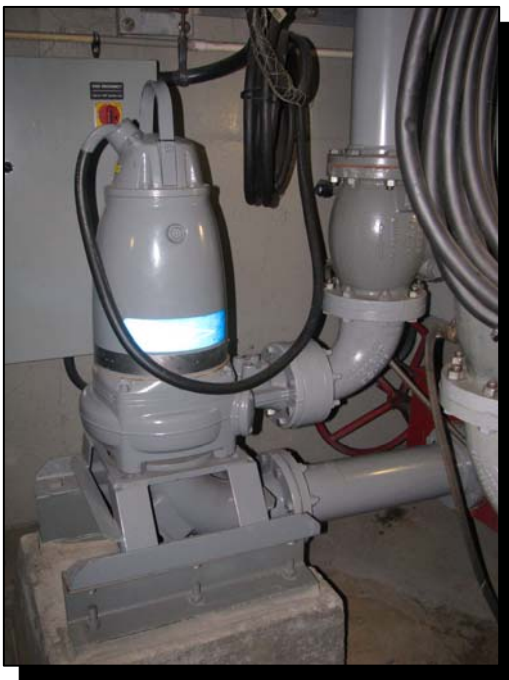
Photograph 6-14 Pacific Avenue Pump Station Pumps
