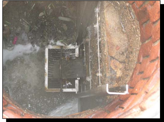
Photograph 6-12 Pacific Avenue Pump Station Wet Well
