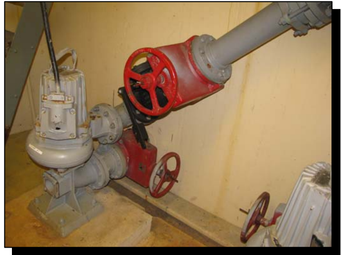
Photograph 6-17 Poinsettia Avenue Pump Station Pumps
