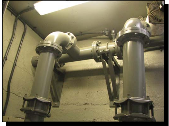
Photograph 6-3 Bell Avenue Pump Station Discharge Header
