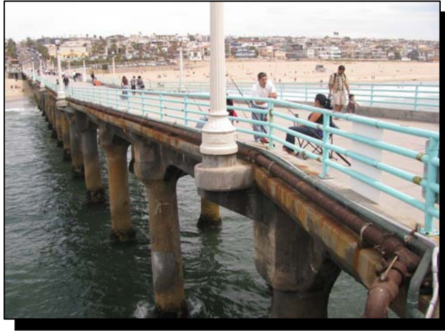
Photograph 6-32 Pier Pump Station Forcemain
