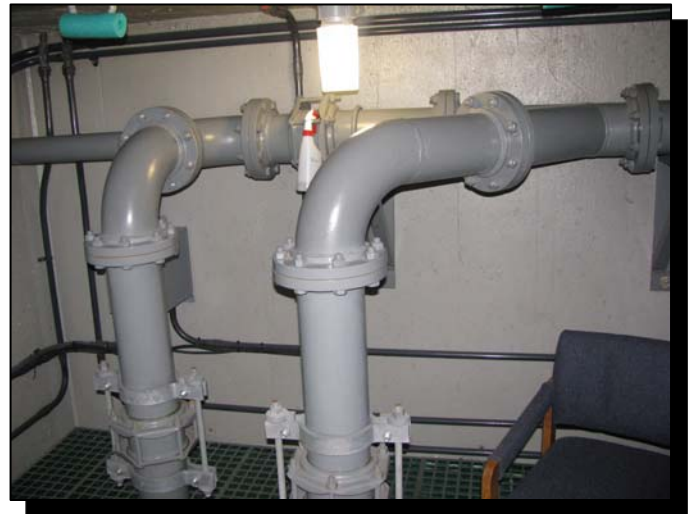
Photograph 6-25 Voorhees Avenue Pump Station Discharge Header
