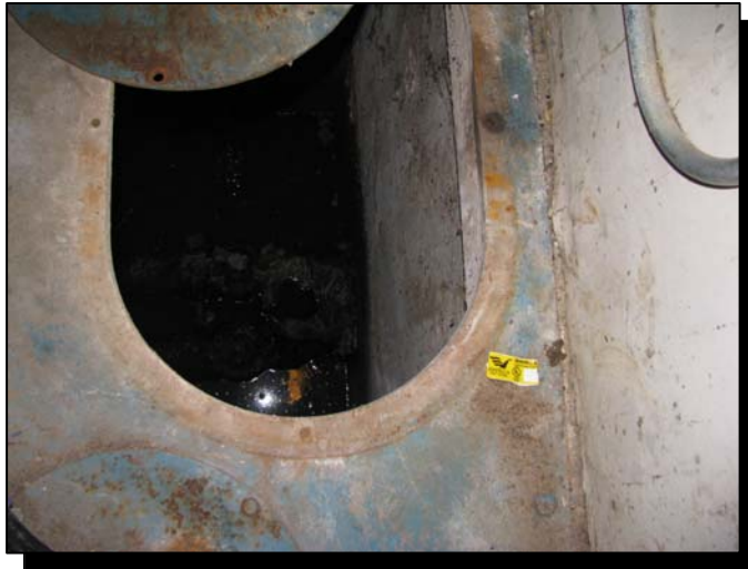
Photograph 6-28 Civic Center Pump Station Wet Well
