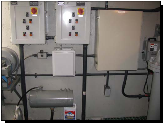
Photograph 6-9 Palm Avenue Pump Station Control Panel
