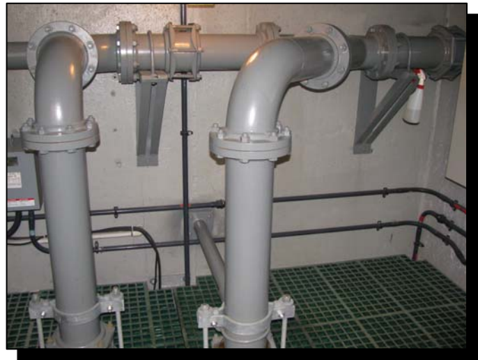
Photograph 6-8 Palm Avenue Pump Station Discharge Header
